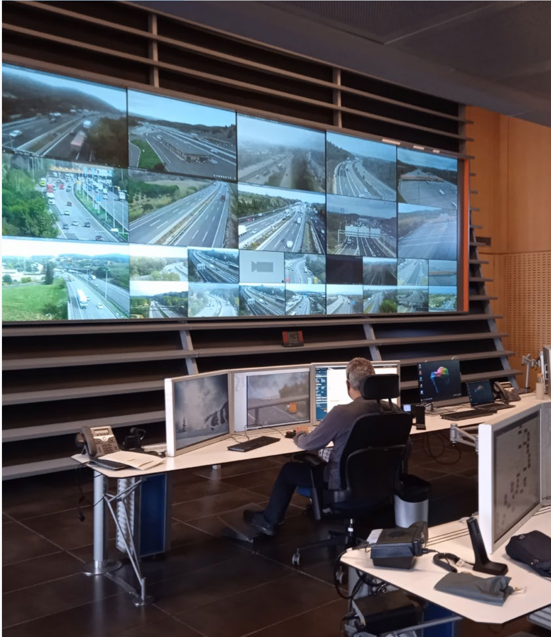
AP-2 and AP-7 Control Center, Granollers (Spain). ►
