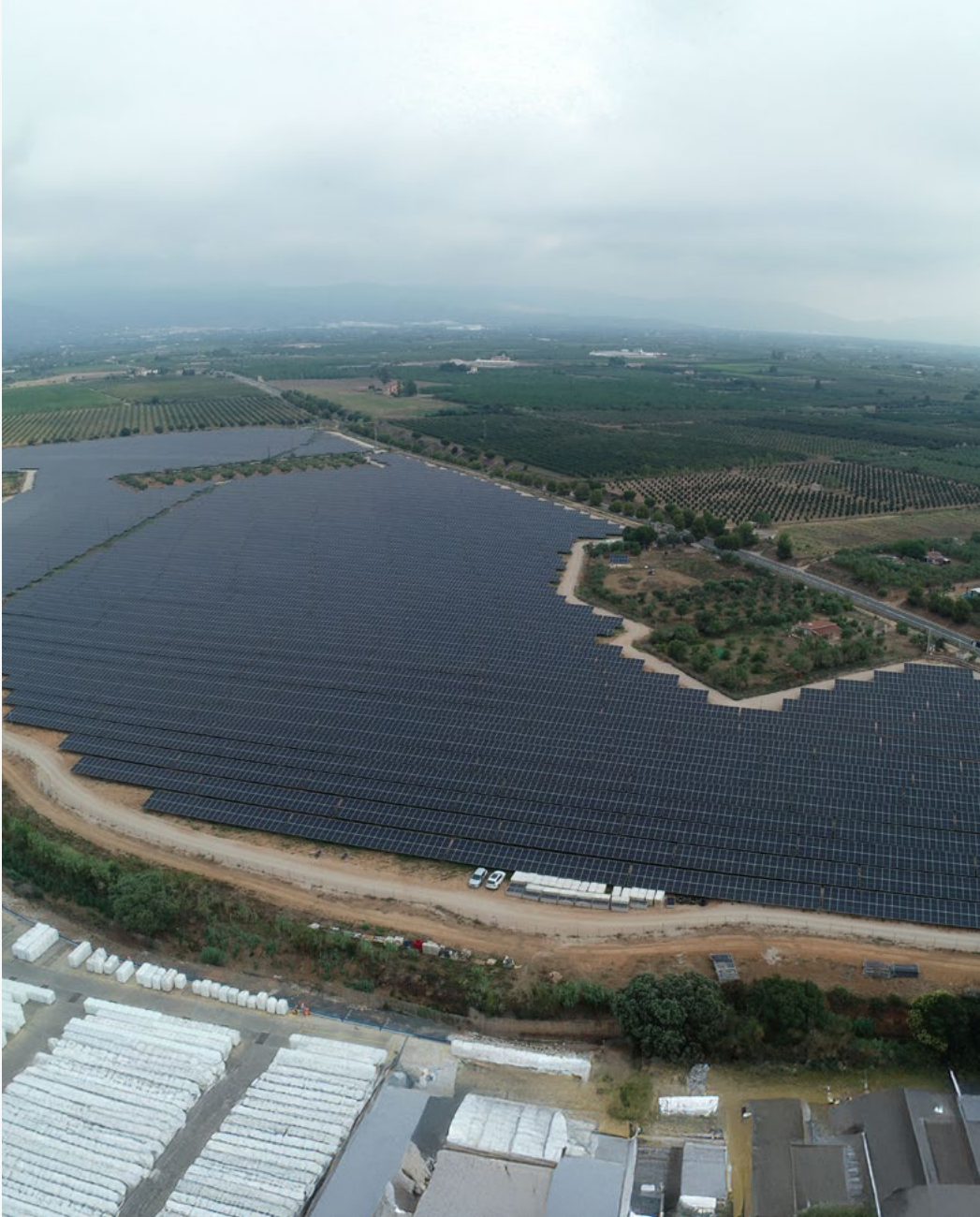
Photovoltaic plant in Constantí, Tarragona (Spain). ▶
