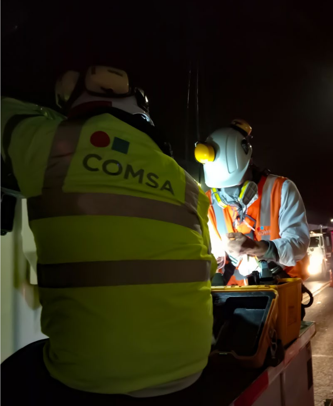
Maintenance of ITS infrastructures in the Sinifaná and Amagá tunnels for the concessionaire Covipacífico, for a period of 10 years (Colombia). ▶
