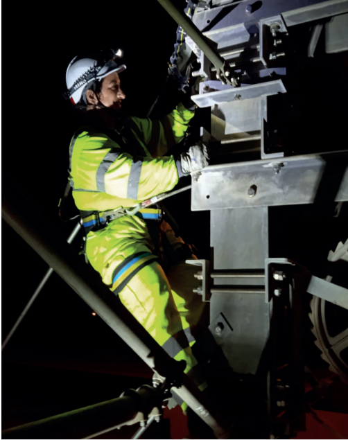
Ana Idáñez, responsible for catenary in the maintenance project for the Alicante tramway.
